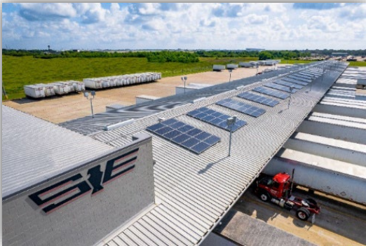
South Houston, TX System Size: 50 kWdc Commissioned in 2013 Net-Metered
