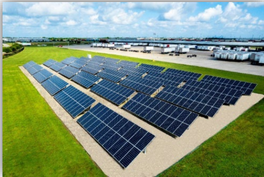
South Houston, TX System Size: 200 kWdc Commissioned in 2013 Net-Metered
