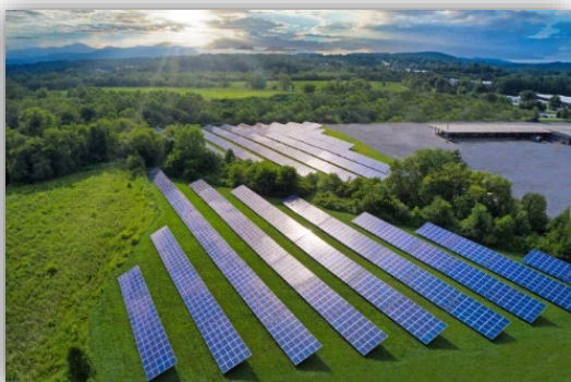
Asheville, NC System Size: 1.2 MWdc Commissioned in 2013 100% Utility Purchased Out of Commission as of Sept 2024 Due to Hurricane Helene
