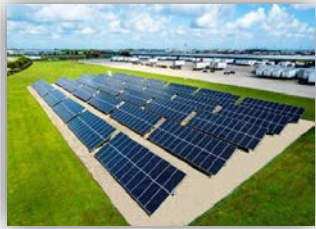
■ South Houston, TX System Size: 200 kWdc Commissioned in 2013
