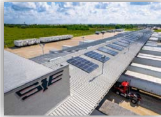
■ South Houston, TX System Size: 50 kWdc Commissioned in 2013
